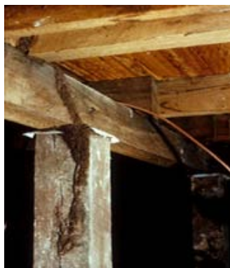
Termite mudding over ant cap.
